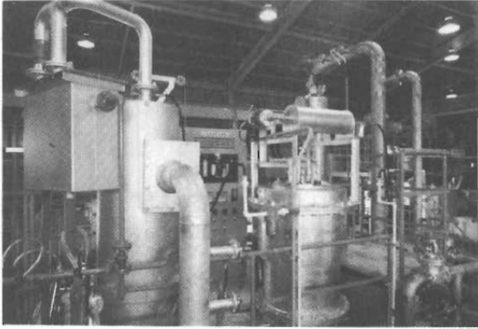
Photo 2 Water-jacket type incineration plant for PVC and rubber wastes
